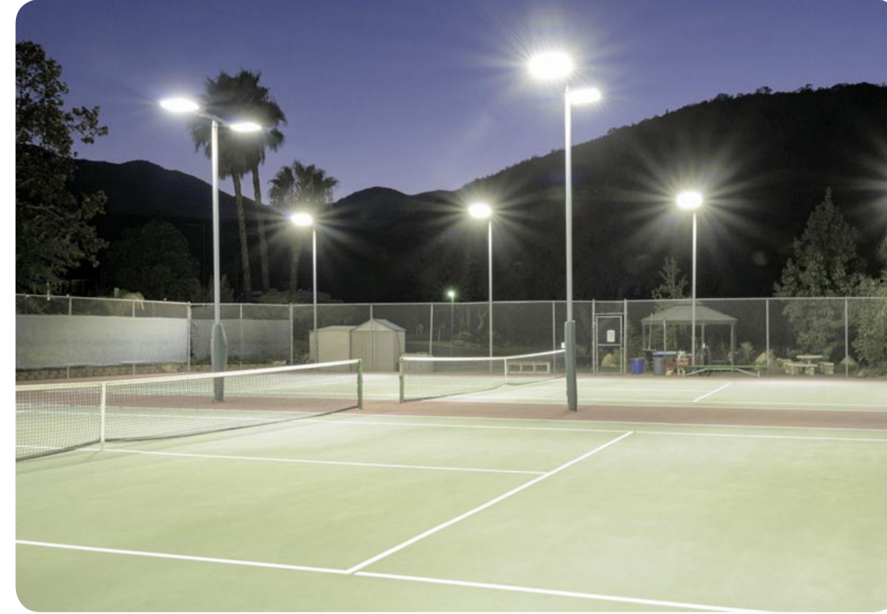
Tennis court lighting
