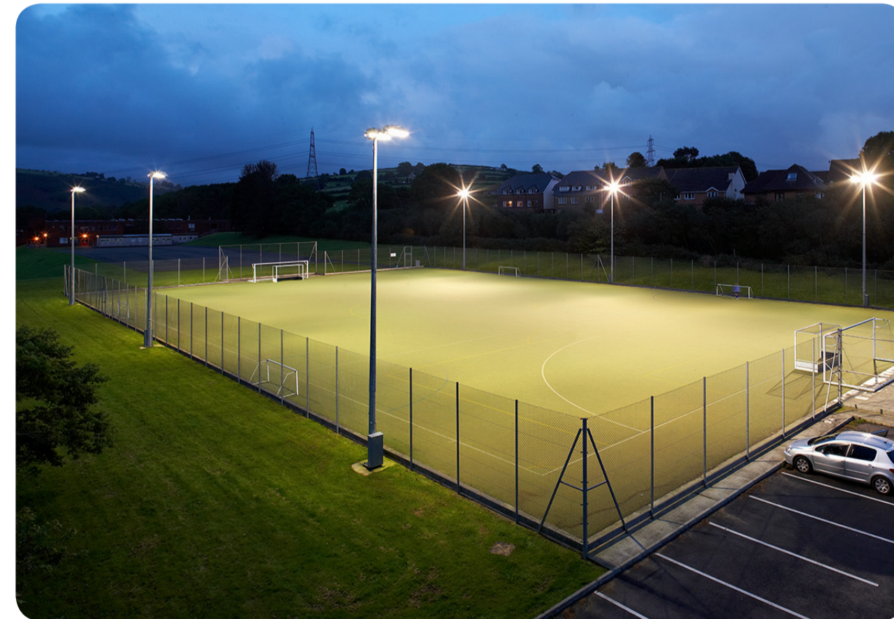
Sporting field flood lights
