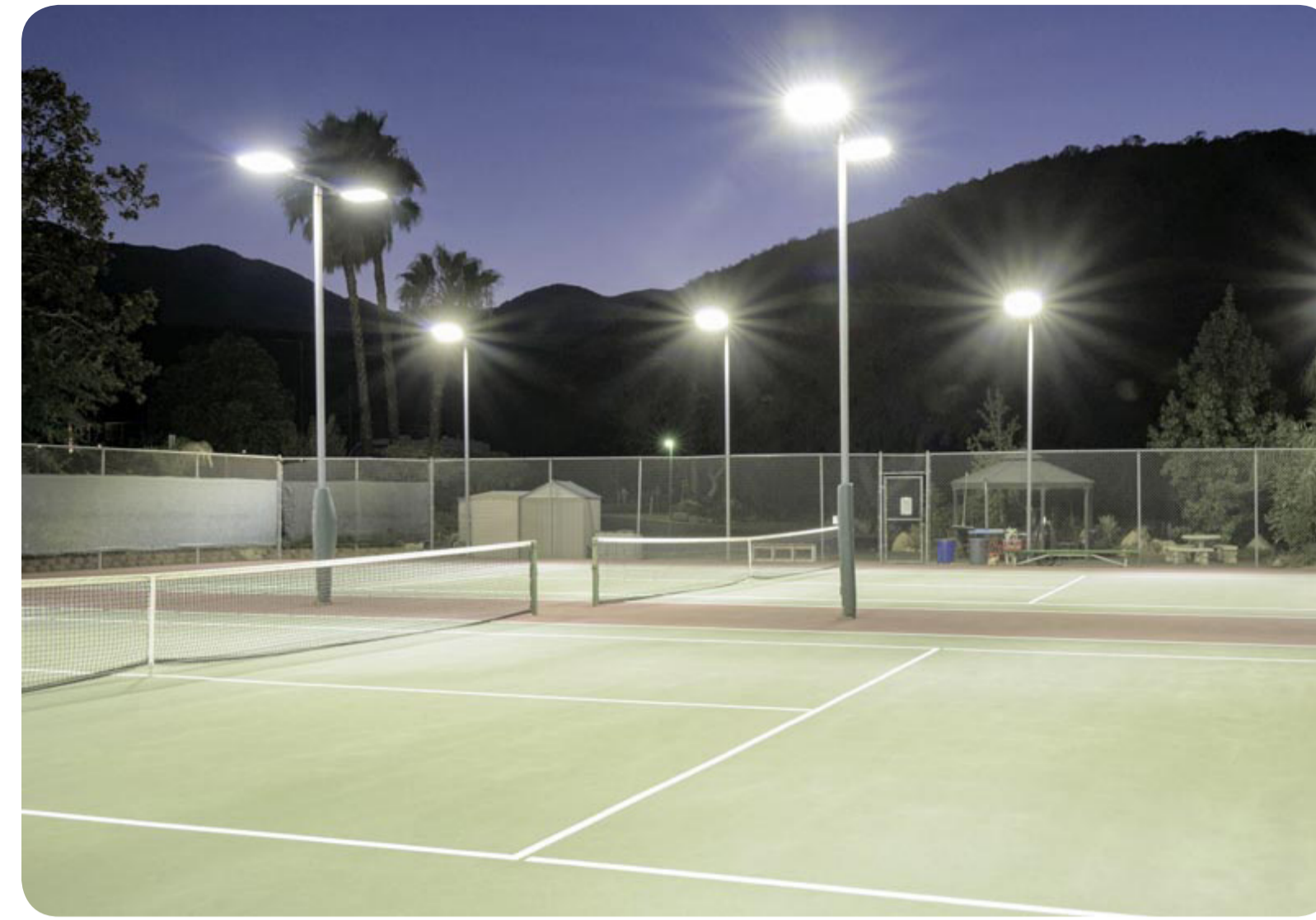
Tennis court lighting
