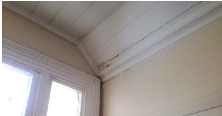
Before project photo: showing internal water damage to ceiling Photo courtesy I. Howse
