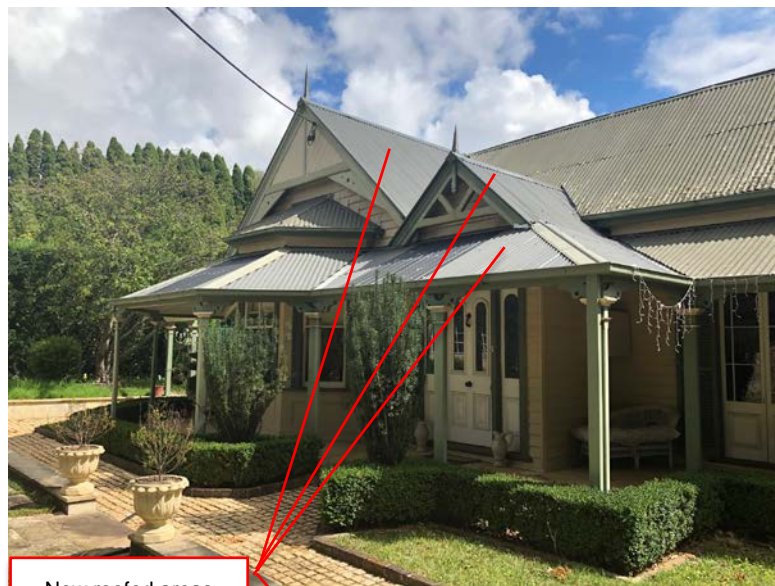
After project photos: Showing side roof repair (left) and rear roof repair (below)
