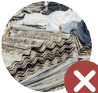
Asbestos or items contaminated with asbestos
