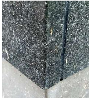
Fig 16: M2 diagonal crack lower front west panel at southwest corner
