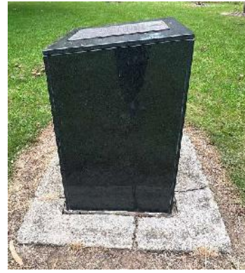
Fig 34: west side with damaged cement footings
