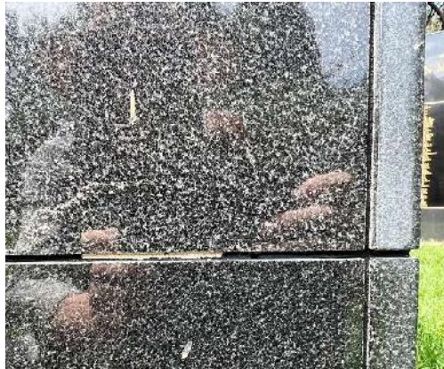
Fig 31: M7 north unpolished grey granite edge and hard white accretion below arc crack above
