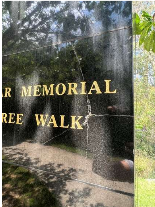
Fig 35: M9 Extensive cracking to obverse inscription panel
