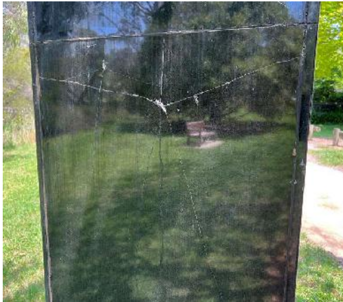
Fig 37: M9 Extensive cracking to north granite panel
