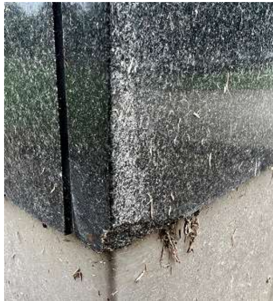
Fig 18: M2 loss at lower southeast corner
