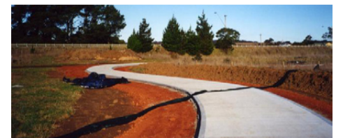
Constructing the Bong Bong track in 2000 (Source: Bong Bong Common Management Committee 2017, http://www.bongbongcommon.org.au/photos/ )
