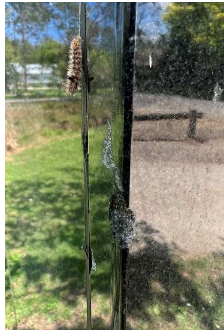
Fig 36: M9 losses to granite on SW edge below cracking on inscription panel
