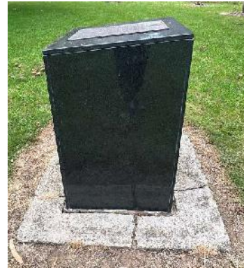
Fig 34: west side with damaged cement footings
