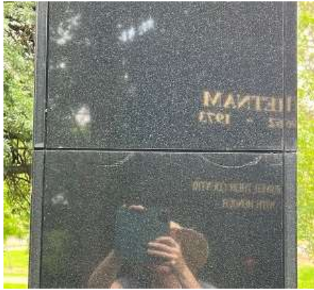
Fig 20: M3 south showing two arc shaped cracks
