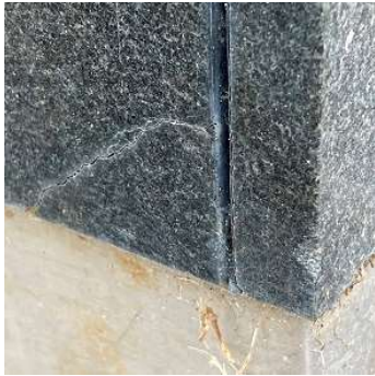
Fig 15: M2 diagonal crack and small loss lower north panel at southwest corner & tea staining on stainless steel skirt at base
