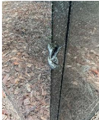
Fig 28: M6 loss on southwest edge and crack on west front facade
