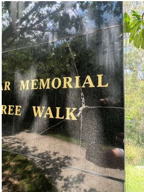
Fig 35: M9 Extensive cracking to obverse inscription panel
