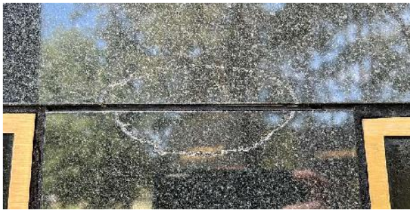
Fig 27: M6 obverse two curved cracks between brass plaques
